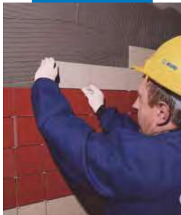
Fixing ceramic tiles on walls working from the top to the bottom
