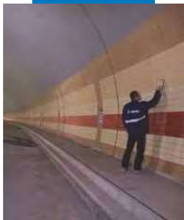
Mrázovka Tunnel - Prague - Czech Republic
